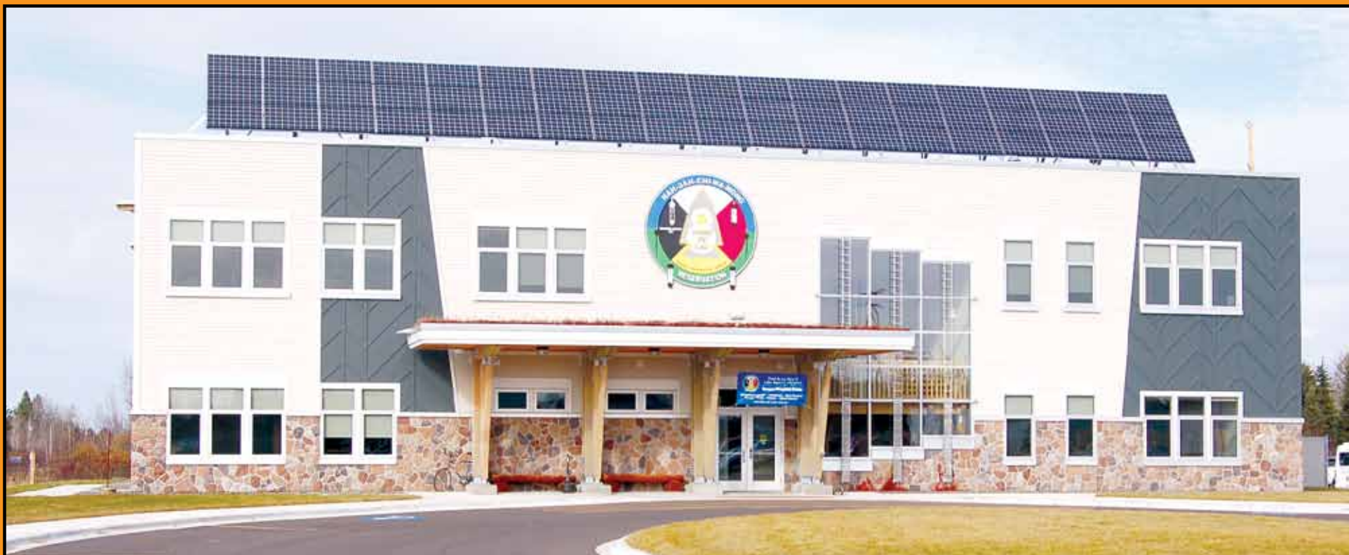
Solar panels were installed to the top of the Resource Management building Oct. 18. The project will be operational within 2-3 weeks, following an inspection of the system and the installation of a new two way electric meter. See story on page six.
