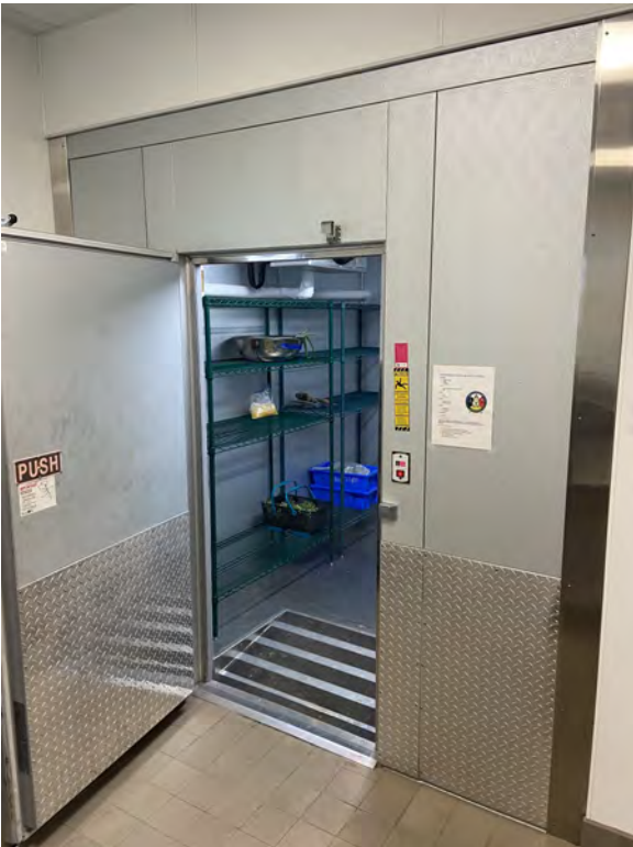
Figure 30. Na'enimonigamig's walk-in cooler , Photograph, taken during site visit.
